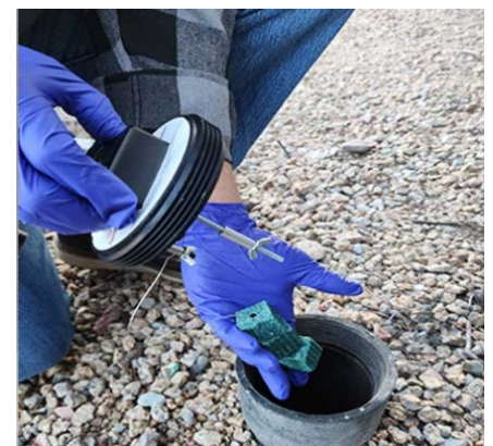
Figure 4: Sewer Assassin in-ground installation
