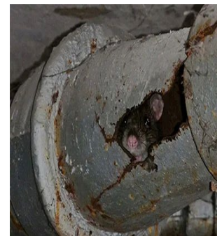
Figure 2: Rat coming out of deteriorated pipe
