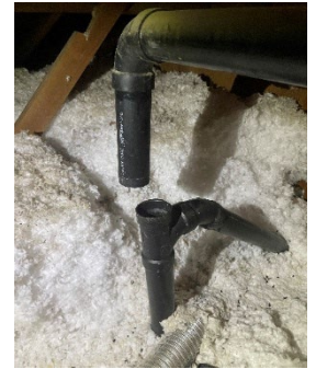
Figure 1: Disconnected Pipe in Attic
