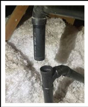
Figure 4: disconnected vent pipe
